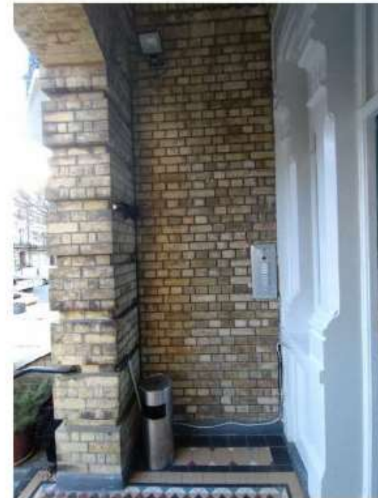
Electrical supply from clients Flat to scooter charging point
